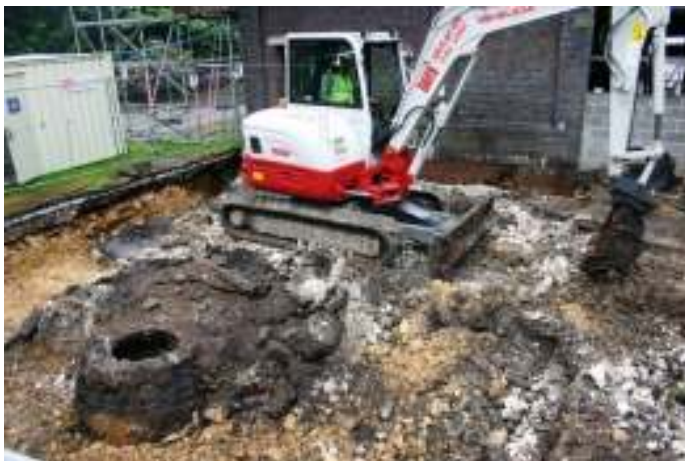
Soon after work started on the foundations for the annexe an old well dug during building in 1889 was uncovered.
