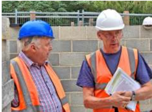
Trustees Stephen Hirst (L) and Will Cook (R) inspect progress of the redevelopment work in summer 2016.
